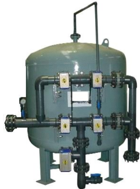
Multi-media filter system
