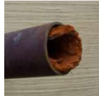
Iron in water causes stains and clogs piping
