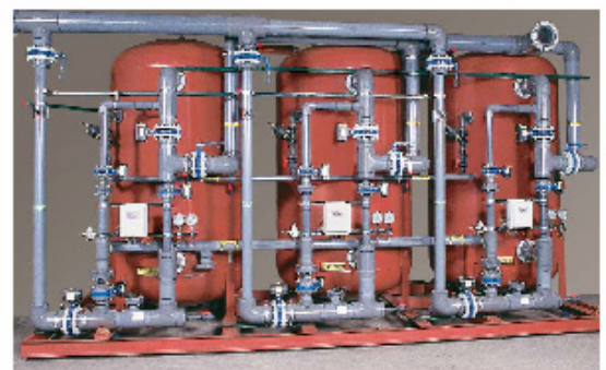
Modern rapid sand filters with automatic backwash systems
